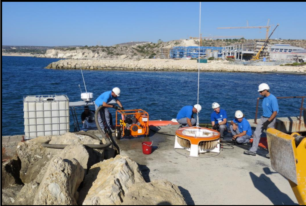
Preparing oil spill response equipment (EAC personnel)
